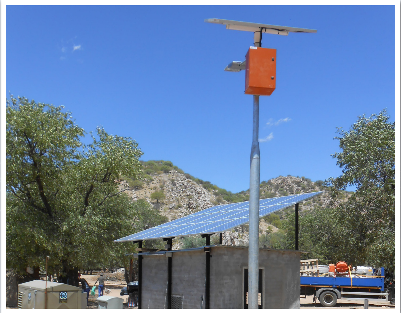
FIGURE 3: KAMDESCHA SOLAR/HYBRID POWER PLANT
